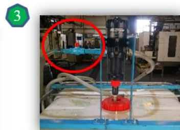
Open the water valve - inlet side to system
