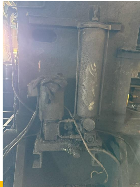
Pumping System & Tank
